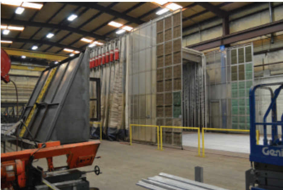
■ Shown here is one of three portable and collapsible paint booths installed by Alfa Laval ACE in 2015. The paint booths are moved into position on tracks built into the floor, allowing coolers to be painted in line without extra handling.
