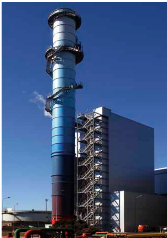
Heat recovery steam generator and chimney
